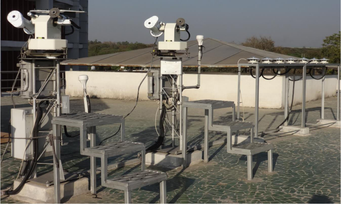
Solar Radiation Calibration Laboratory (SRCL) at NISE Surya Bhawan.
